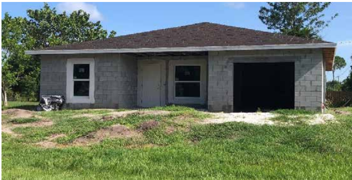
NW Sherbrooke Ave: Ready for drywall and exterior finish after June's SLC School's Vocational Program Students.
